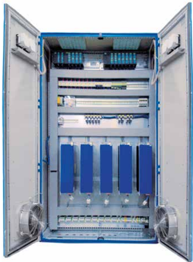
The ELC® Power Supply Unit installed in the switch cabinet.
